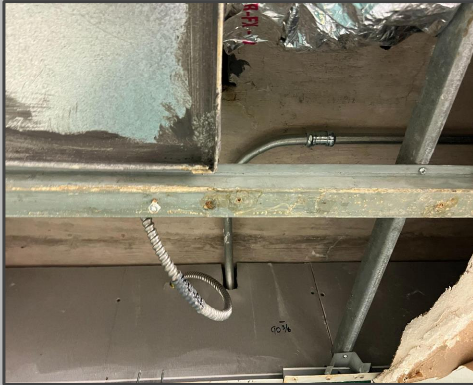
Exposed roofing/damaged ceiling tiles near staff lounge
